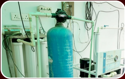
RO Water Plant
